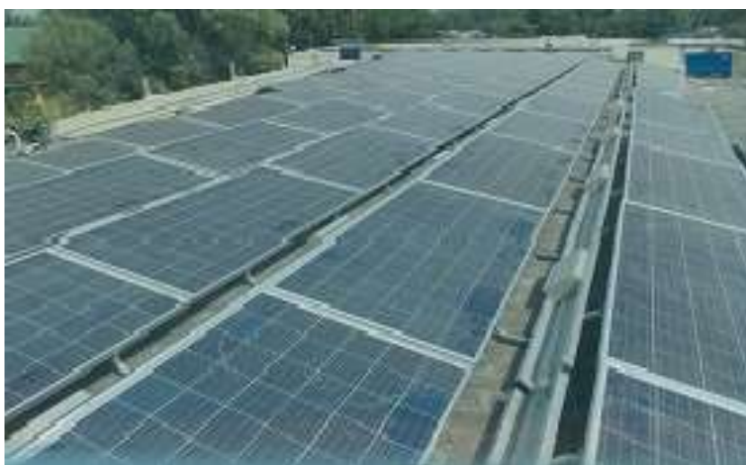
Fig. Solar power plant installed in the SLC campus
